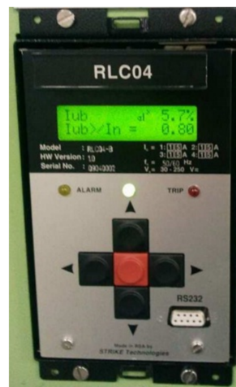
Figure 6: Current unbalance level after commissioning
