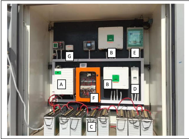
Fig. 4. Installed PV power solution for an off-grid rural bakery. Battery inverter (A), PV inverter (B), battery bank(C), PV charger (D), PV switching panel (E), AC distribution board (F), system monitor (G).
