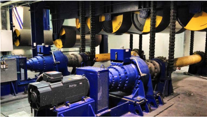
Figure 4. Drives of the looper car on a real continuous line
