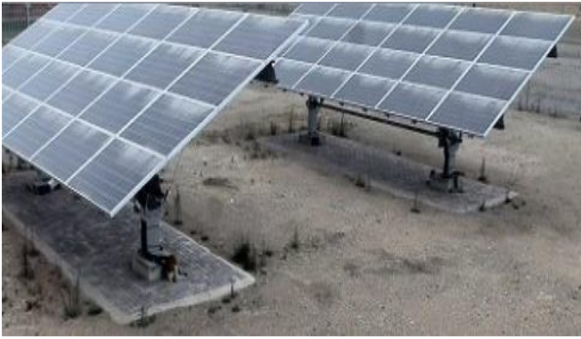
Figure 2: Pilot PV system with single-axis solar tracking installed in Limpopo, South Africa
