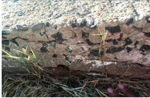
Figure 1 Disintegrated concrete weir at a site of acid mine drainage decant (Azene & Ekolu 2012)
