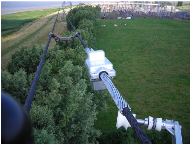
Fig. 2. Ampacimon installation on a 400 kV line [21]
