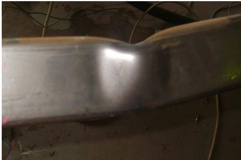
Figure 11 Inward distortional buckling
