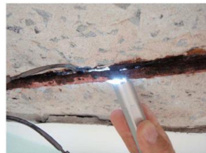
Figure 3 Severely corroded bar, completely debonded from concrete
