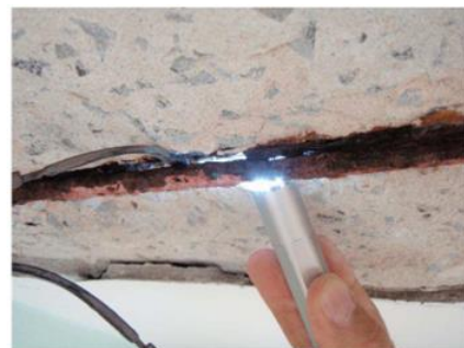
Figure 3 Severely corroded bar, completely debonded from concrete
