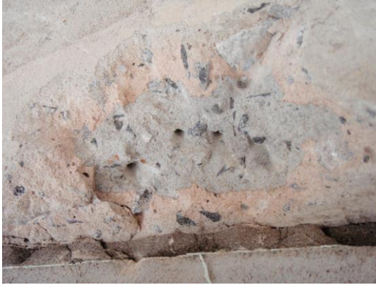
Figure 4. Field evidence of colour change (to orange) in the outer layer of concrete compared to the original gray colour seen in the interior concrete
