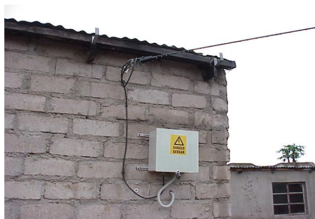
Fig. 4 Service cable entering the house-hold
