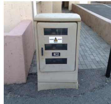
Fig.1 Customers distribution box
