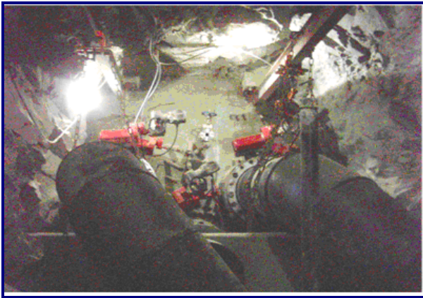
Figure 7: 27 level plug valve at Kloof 10 shaft
