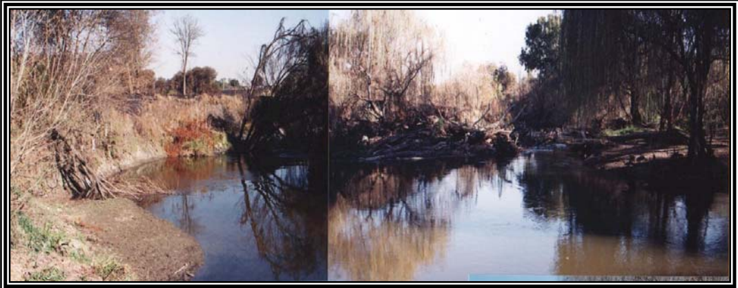
May 1998, downstream view (note eroded banks).
